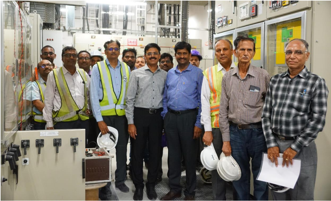
Image 3 - Mr. DVS Raju and Mr. KVB. Reddy, along with officials from HMRL, L&TMRHL & AECOM (Concessionaire Engineer) at Chikkadpally ASS
